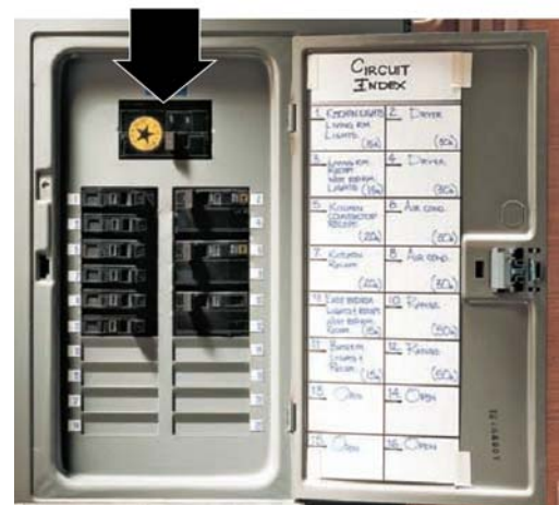
Main Circuit Breaker
